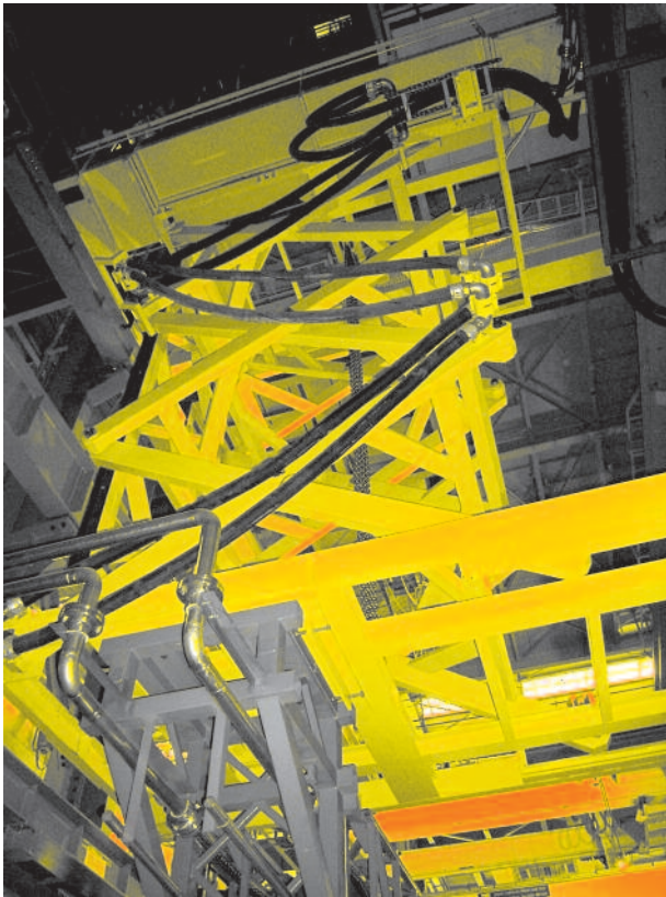
Lifting system at pantograph Applied at crane
